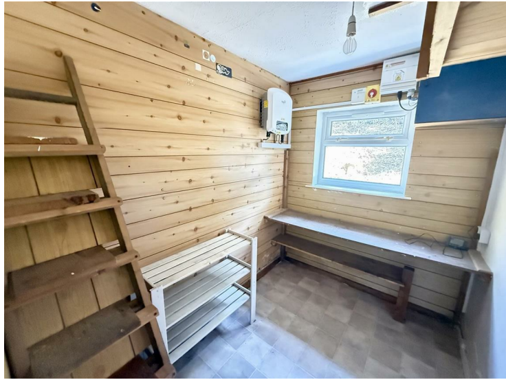
A useful room with the solar panel equipment
